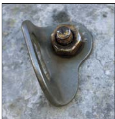
Corroded Rocklands bolt - DANGEROUS!
